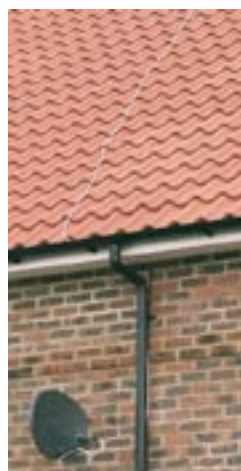
A not so good example, where an obvious white lead has been trailed across the roofline.
